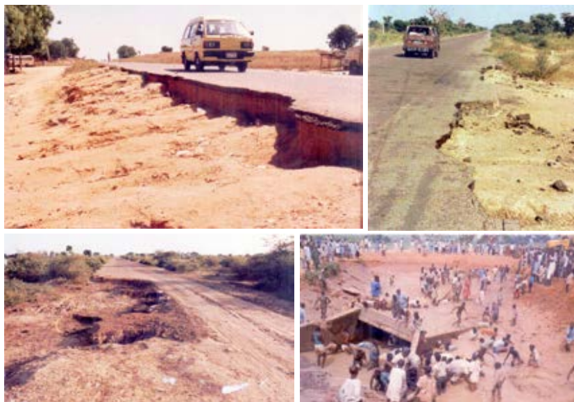
Figs. 1 – 4: Typical road failures
