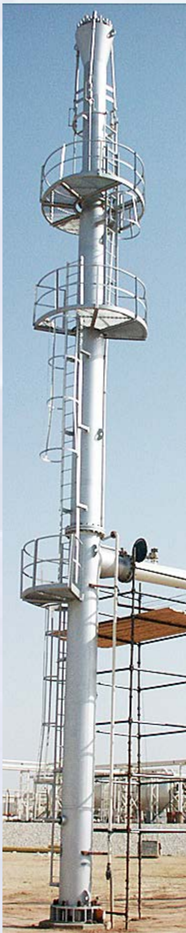
Boskel's Smokeless Flare System installed in Oman
