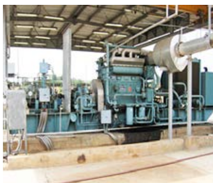
Fig. 2: Diesel Driven Mainline Pump
