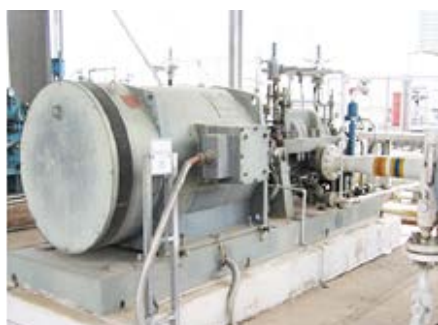
Fig. 3: Electric Motor Driven Mainline Pump
