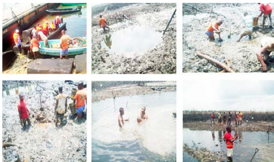
Figs. 8, 9, 10, 11, 12 &amp; 13: Vandalized pipelines maintenance efforts by NNPC
