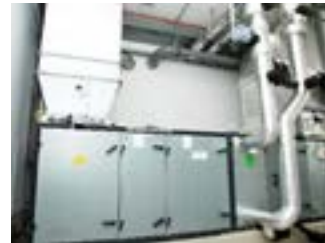
Air handling units installed at PTDF Head Office, Abuja
