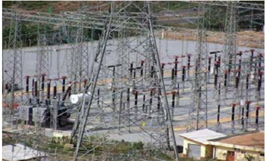
Fig. 1: The Katampe Substation, Abuja
