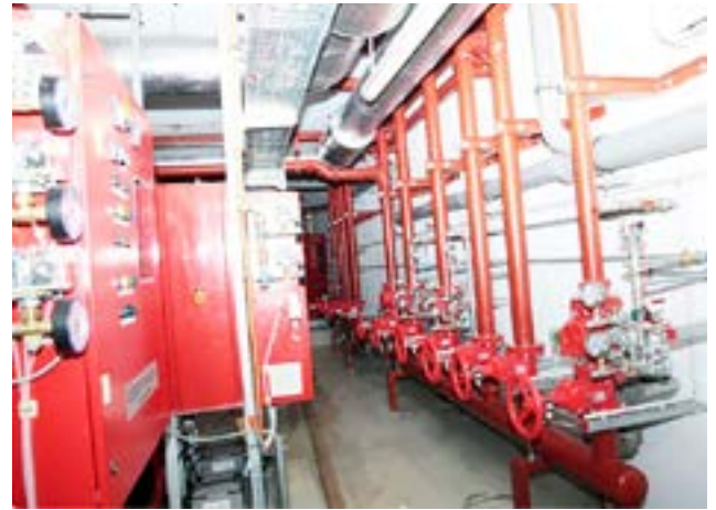
Fire pumps installed at PTDF Head Office, Abuja
