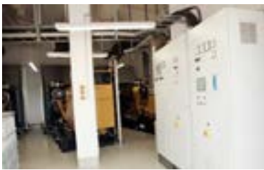
Generators installed at PTDF Head Office, Abuja
