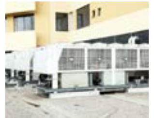
Chillers installed at PTDF Head Office, Abuja
