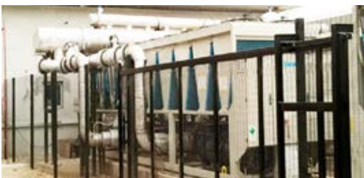
Chillers installed at NCDMB Head Office, Bayelsa State
