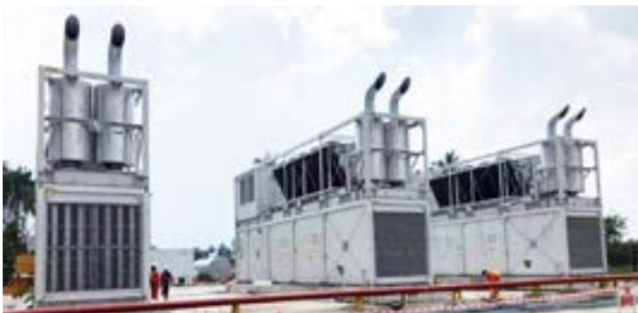
Generators installed at NCDMB Head Office, Bayelsa State
