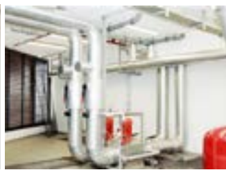
Pumps installed at PTDF Head Office, Abuja
