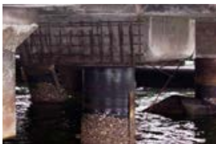
Fig. 4: An exposed rebar
