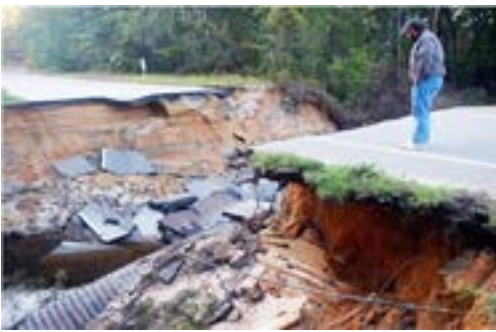
Fig. 2: Road pavement erosion
