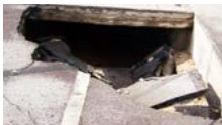
Fig. 3: Pavement caving in
