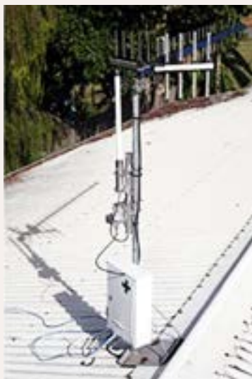
Fig. 10: A rooftop 1 watt Wi-Fi amp, feeding a simple vertical antenna on the left
