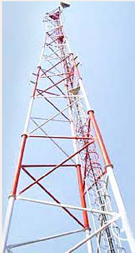
Fig. 1: A telecoms mast
