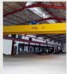
CUMMINS WEST AFRICA, LAGOS 20 Tons DEMAG Crane Completed 2020
